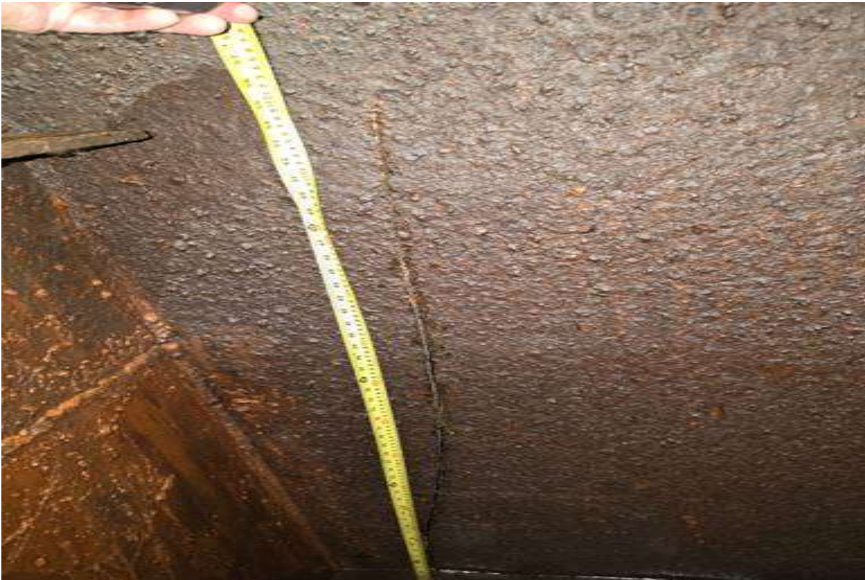
Figure 4. 55-inch crack in the longitudinal bulkhead.
